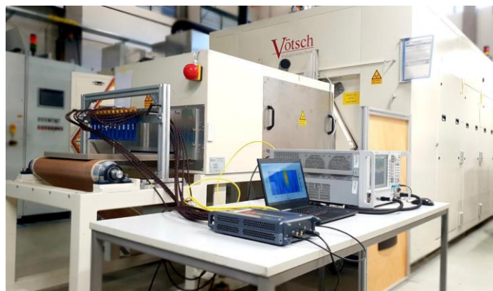
Fig. 37: The MWT sensor installed at the inlet of the HEPHAISTOS oven
